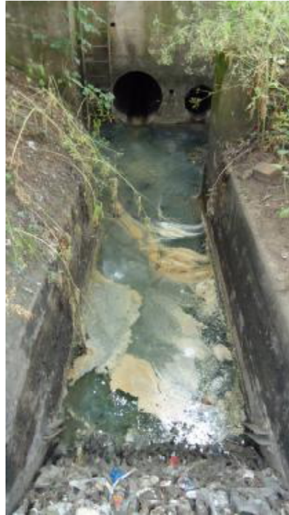
The Wharf Brook at the discharge point and end of the culvert in the western section of the site
